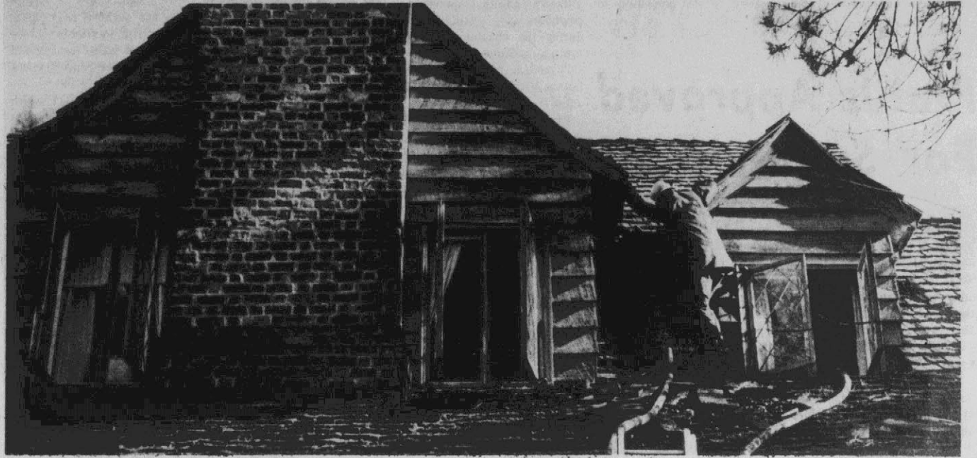
HOME DAMAGED BY FIRE . . . The Alton Barrett home at 517 Longmeadow Rd., was heavily damaged by fire yesterday. Above a Greenville fireman makes his way across the roof of the home after fire caused heaviest damage to the second floor, and smoke and water damage to the lower rooms. (Reflector Photo by Tommy Forrest)
