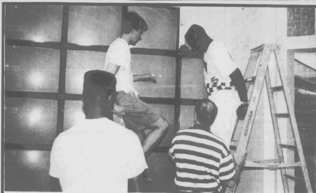
Last Minute Details - Belk at The Plaza... Technicians and workmen are shown installing the 16 television bank at the Arlington Boulevard entrance of the new 46,000 sq. ft. Belk store. MTV entertainment tapes will be played on these units. The store will open Wednesday, July 26, with a ribbon cutting ceremony to begin at 9:30 a.m. Refreshments and entertainment will be provided beginning at 8:45 a.m.
