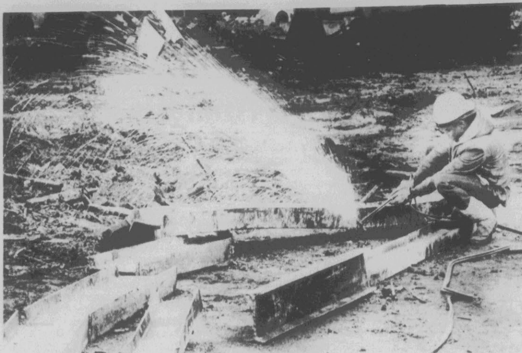
SPARKLING JOB — Arthur Jackson uses a torch to cut through steel at the site of a new hotel-shopping complex in Durham, sending up a shower of bright sparks.
