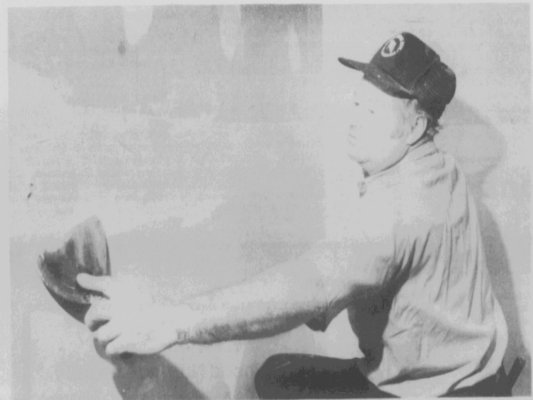
ADDING OFFICES — Public Works Department employee Tom Stencil uses joint compound to finish sheet rock inside City Hall. He is part of a crew building new office space inside the municipal building. (Reflector Photo by Cliff Hollis)
