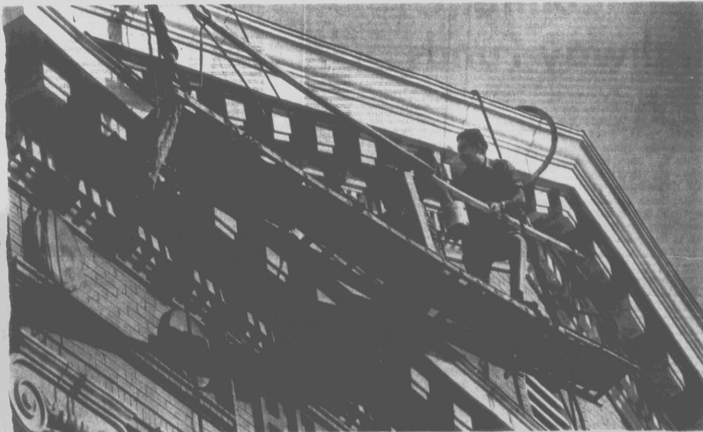
FRESH PAINT — Workmen on high-rise equipment take advantage of warmer weather to give the Pitt County Courthouse a fresh coat of exterior
