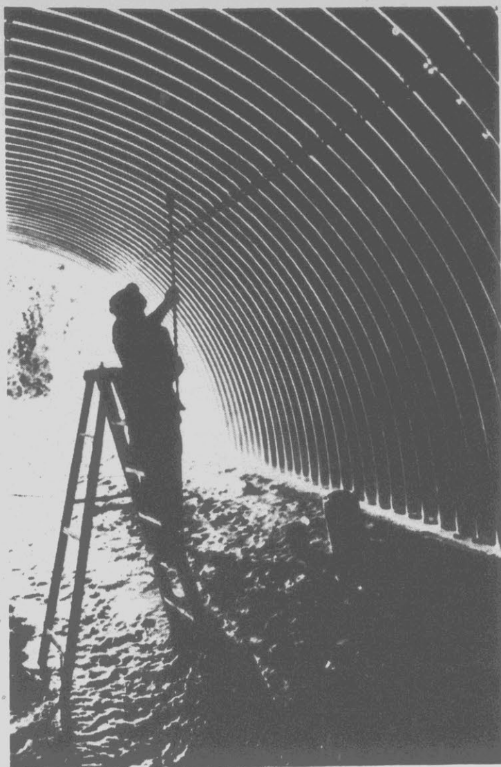
TUNNEL VISION — Sometimes your work can produce more than you bargained for, and that may be the way worker Darwin Morrow feels as he works on the inside of this culvert. He was painting the aluminum culvert under Henry Street in Spartanburg, S.C. (AP Laserphoto)
