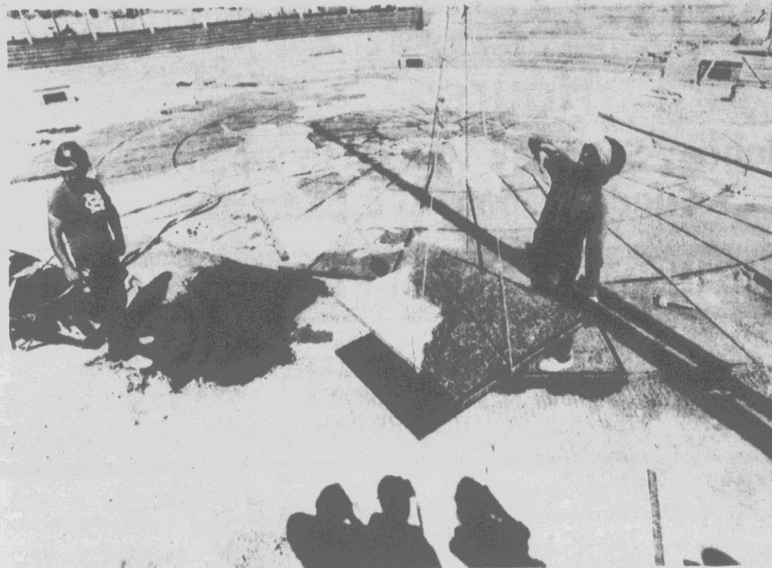
WORLDLY WORK — Workmen lower a granite section of what will be part of a circular plaza 100 feet in diameter. The plaza will bear a grid map of the United States at the U.S. Navy Memorial in Washington. The
