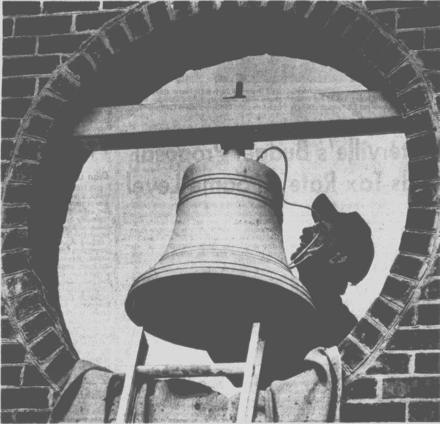
SCHOOL BELL INSTALLED — Workman Jeff Smith installs the clapper of a 200-pound bell at the new Pitt County elementary school near Bells Fork. The bell was donated to the school by local architect James Hite, who was the
