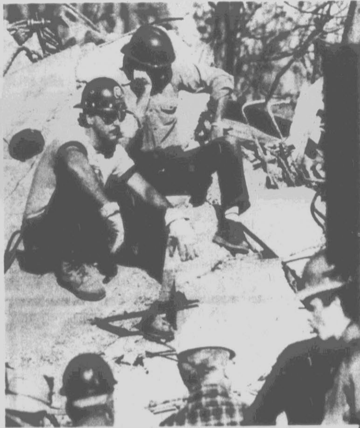
TAKING A BREAK — Weary rescue workers take a break as around-the-clock digging continues in the rubble of an apartment building that collapsed in Bridgeport, Conn., last Thursday. Fifteen workers are still missing in the collapse, which killed 13 other workers. The first funerals for victims of the accident were scheduled today. (AP Laserphoto)
