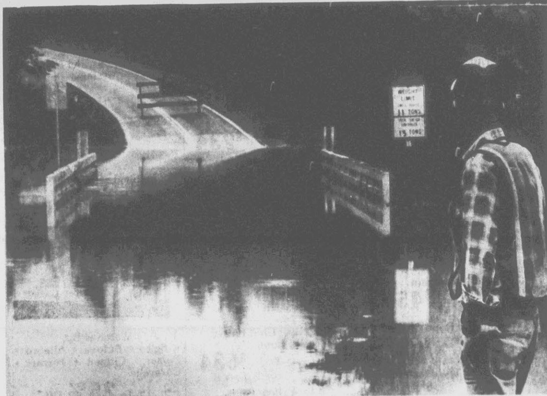
BRIDGE FLOODED — A.E. Moore, a Department of Transportation maintenance supervisor in Alamance and Orange counties, looks at the rising water of Beaver Creek near Alamance as it crosses a highway bridge.
