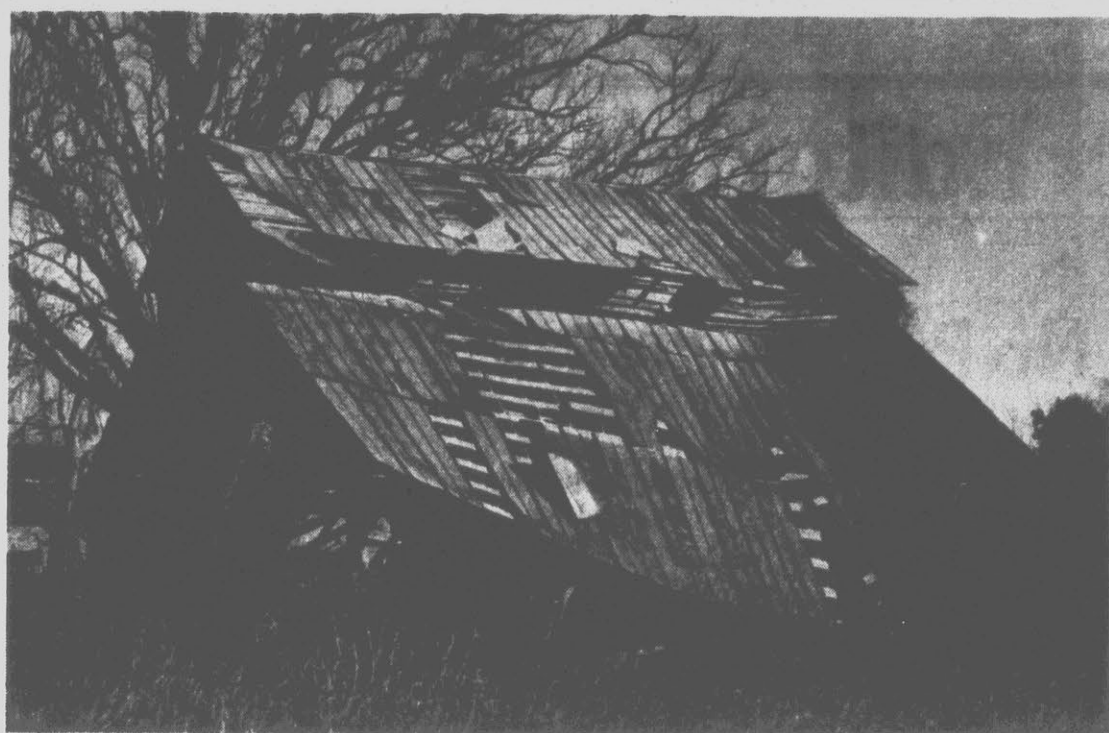
ANOTHER WINTER — An abandoned barn at an unoccupied Pitt County homestead has survived another winter and stands solid except for torn-away sections of the upper and shelter roofs that expose the barn's framework. This barn design, popular some years ago, features a long sloping roof that saved on building expenses while at the same time providing additional one-story storage space adjacent to a two-story main structure. (Reflector Photo by Jerry Raynor)
