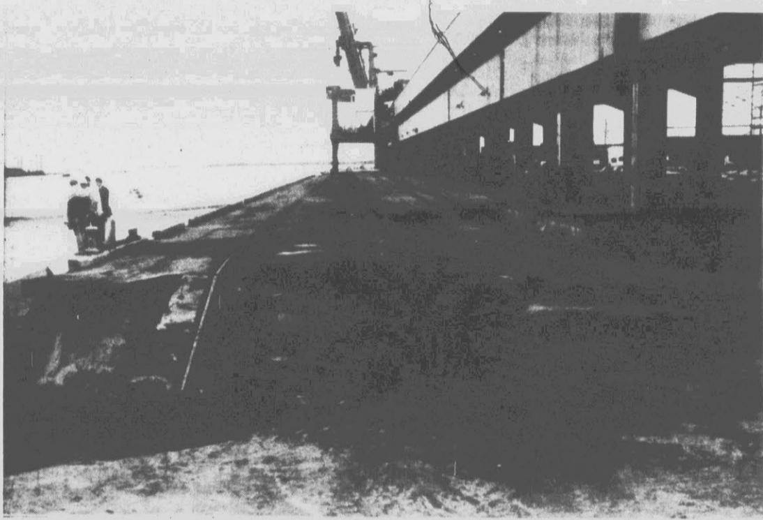
BERTH DAMAGED — Erosion sparked in part by offshore dredging buckled railroad tracks, sideswiped a supply store and threatened to dump thousands of gallons of oil from tanks being emptied by emergency crews at the Morehead City port, officials said. (AP Laserphoto)
