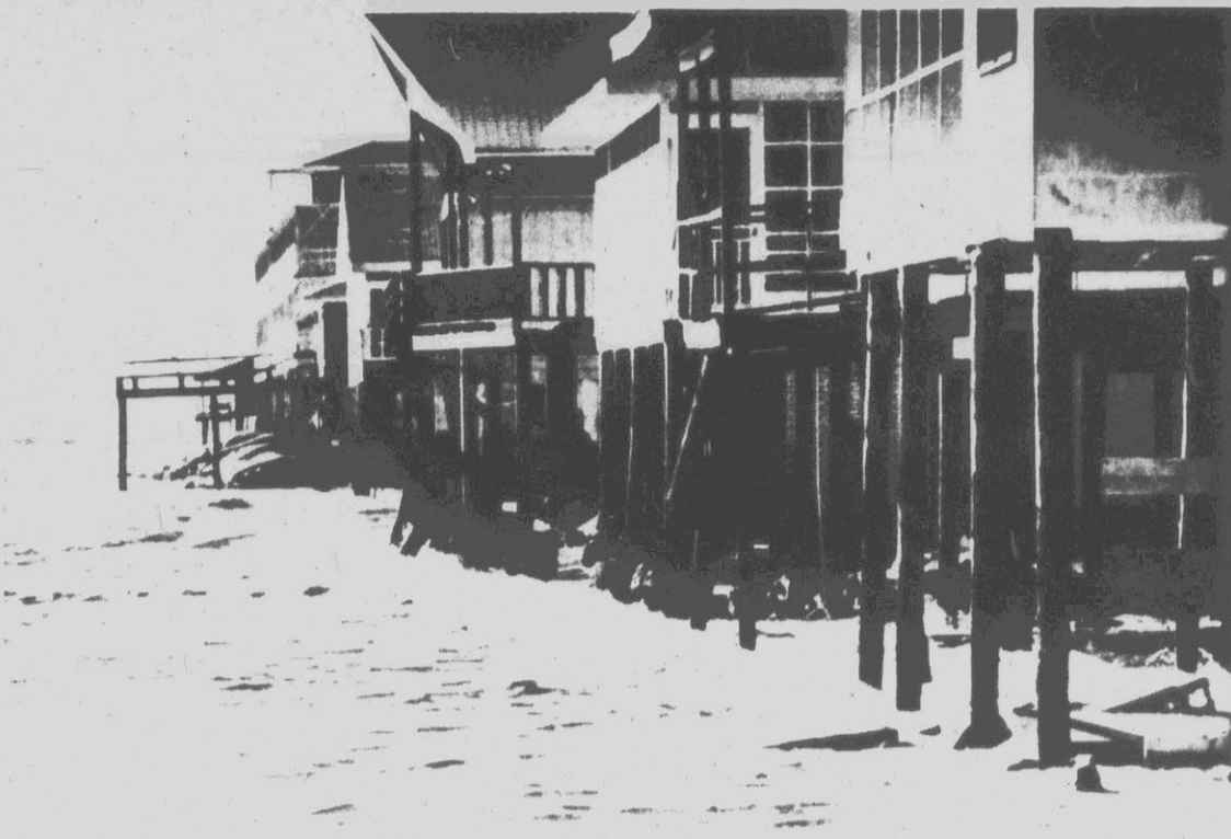
OCEAN FRONT — While some people dream of having ocean front property, the owners of these cottages at Topsail Island probably wish otherwise. Without any natural
