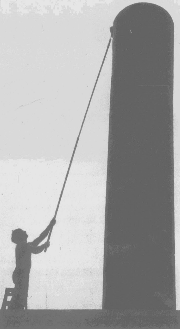
STACK PAINTING — Most of us try our hand at painting at one time or another, but it isn't always that easy. An East Carolina University maintenance worker uses a long pole and a roller to paint a smoke stack on the East Carolina steam plant on a recent afternoon. (Reflector Photo by Chris Bennett)
