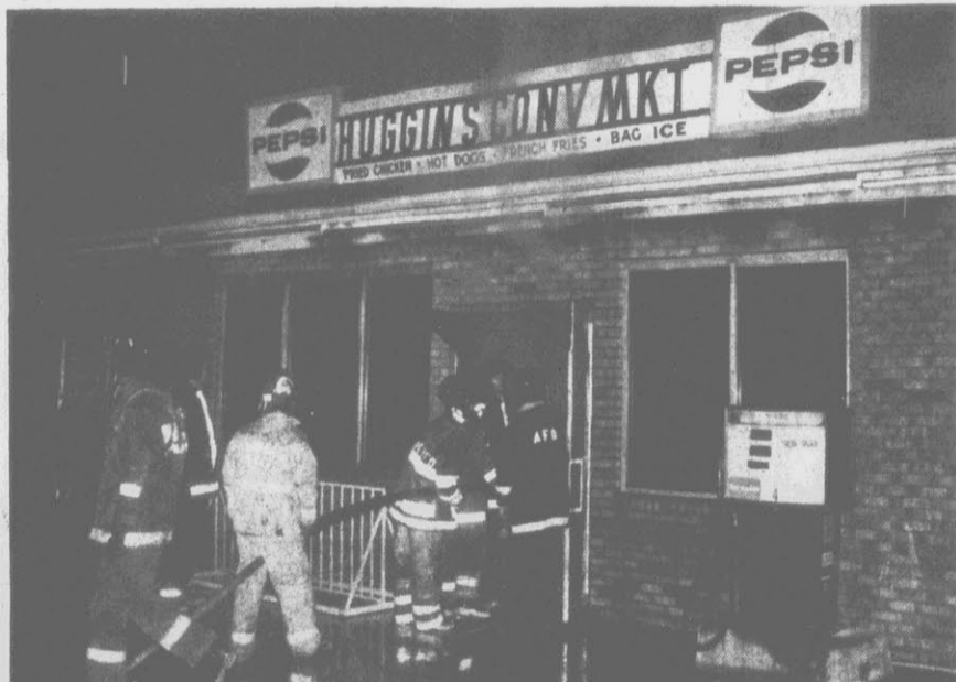
BLAZE DAMAGES AYDEN BUSINESS — Fireman battle an early-morning blaze that county fire officials say heavily damaged Huggins Convenient Mart and Laundromat on South Lee Street in Ayden today. Pitt County Fire Marshal Bobby Joyner said no dollar estimate of damage was available and that the cause of the fire is under investigation. Two Ayden
