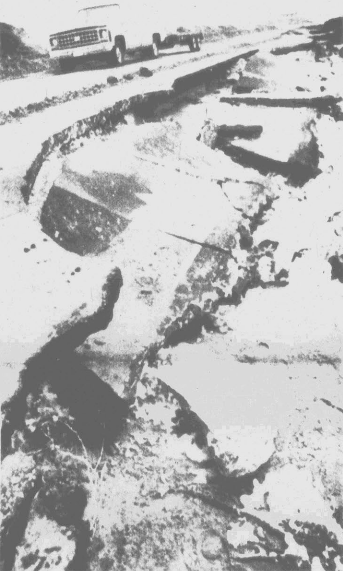
STORM DAMAGE — A pickup truck drives past a washed out portion of Caswell Drive after wind-whipped seas cut into the Creswell Beach road Tuesday. Some authorities say erosion on the coast was worst Tuesday and today than from Hurricane Diana. (AP Laserphoto)
