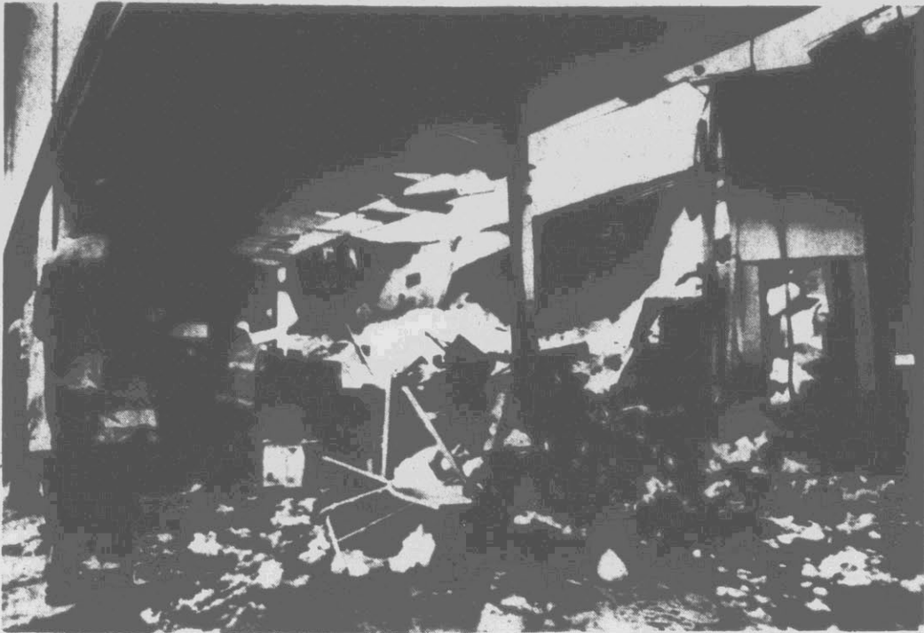
ROOF COLLAPSE — Volunteer firemen survey the scene of the Mills department store in the Buffalo, N.Y., suburb of Clarence where a large section of roof caved in under the weight of too much snow Sunday. Nine people were taken to area hospitals where only minor injuries were reported. (AP Laserphoto)
