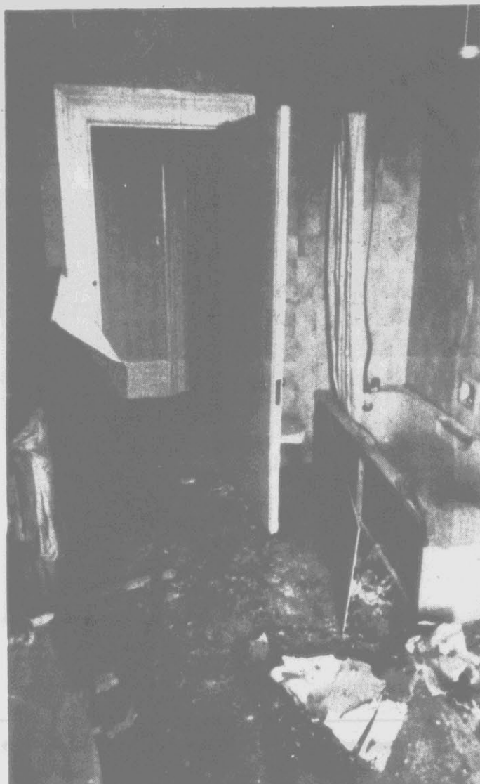
SHATTERED BATHROOM — Britain's Prime Minister Margaret Thatcher's bathroom in the Grand Hotel Brighton, Brighton, England, is shown Sunday following the IRA bomb blast Friday. Premier Thatcher had left her bathroom on her first floor suite two minutes before the blast occurred five floors up. (AP Laserphoto)
