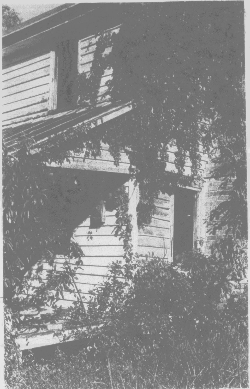
ENCROACHMENT — Once a building is no longer tenanted, nature loses no time in its relentless encroachment of an unguarded structure on which it can spread its web of covering vines.
