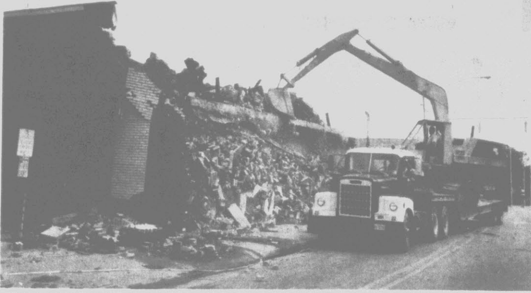
FRONT WALL FALLS... Construction equipment was used to bring down a portion of the front wall of The Attic following an early Sunday morning fire at the nightclub. The photo above shows the upper portion of the wall as it falls to the sidewalk. (Reflector Staff Photo).
