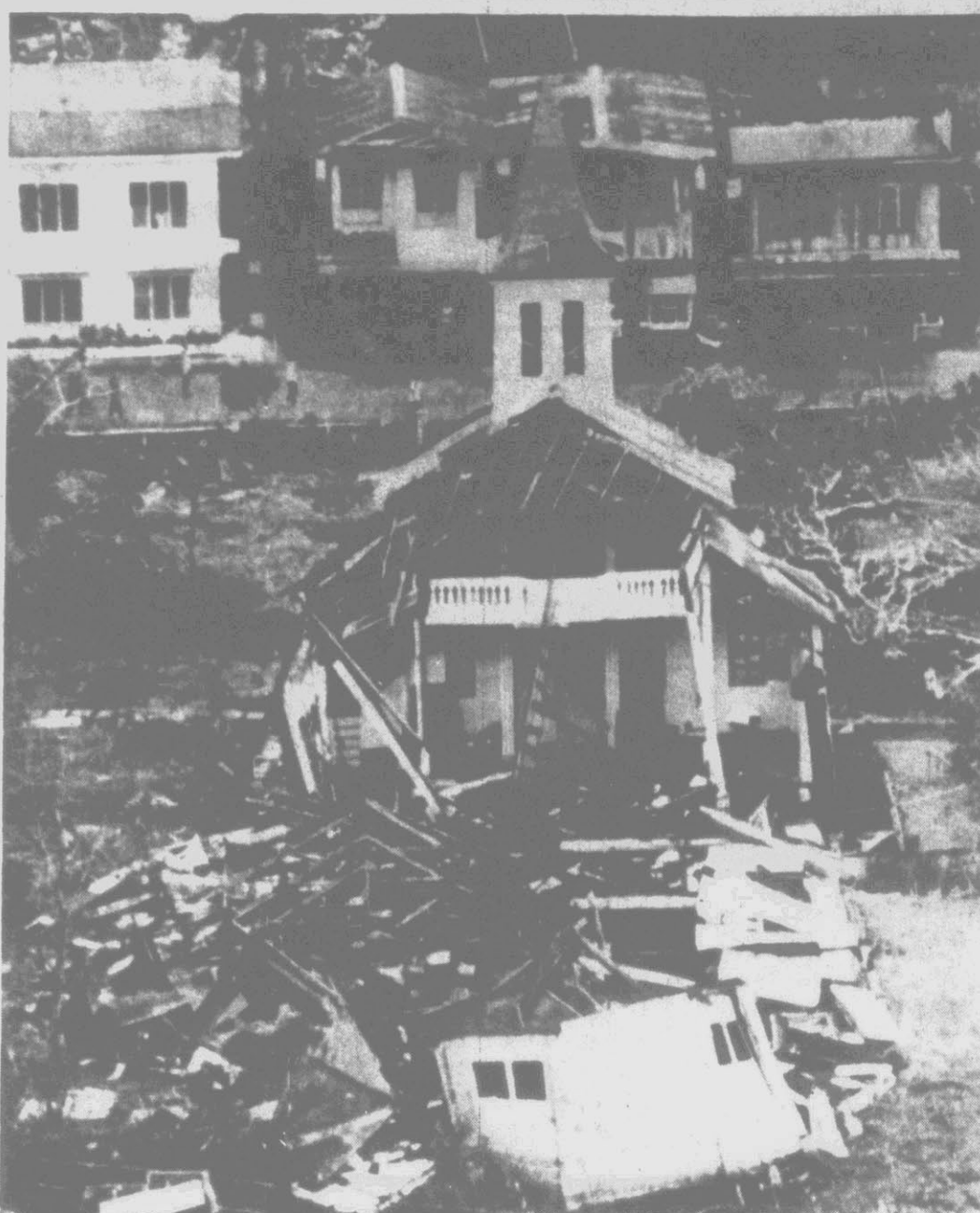
TYPHOON DAMAGE — Only the steeple shows that the collapsed building above is a church, one of the thousands of houses and buildings shattered by Typhoon Ike's 115-mph winds in the Philippines. The church was located in Suricao City, about 450 miles south of Manila. More than 1,000 people died and 200,000 others were left homeless in the typhoon's wake. (AP Laserphoto—
