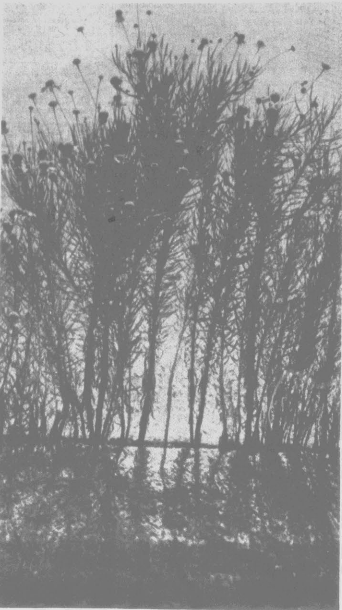
ROOT POWER — The astonishing power of roots to break through any surface is demonstrated by this line of common sneeze weeds. The ferny, yellow-blossomed weeds cracked open an apron of concrete to seek sun and air. (Reflector Photo by Jerry Raynor)
