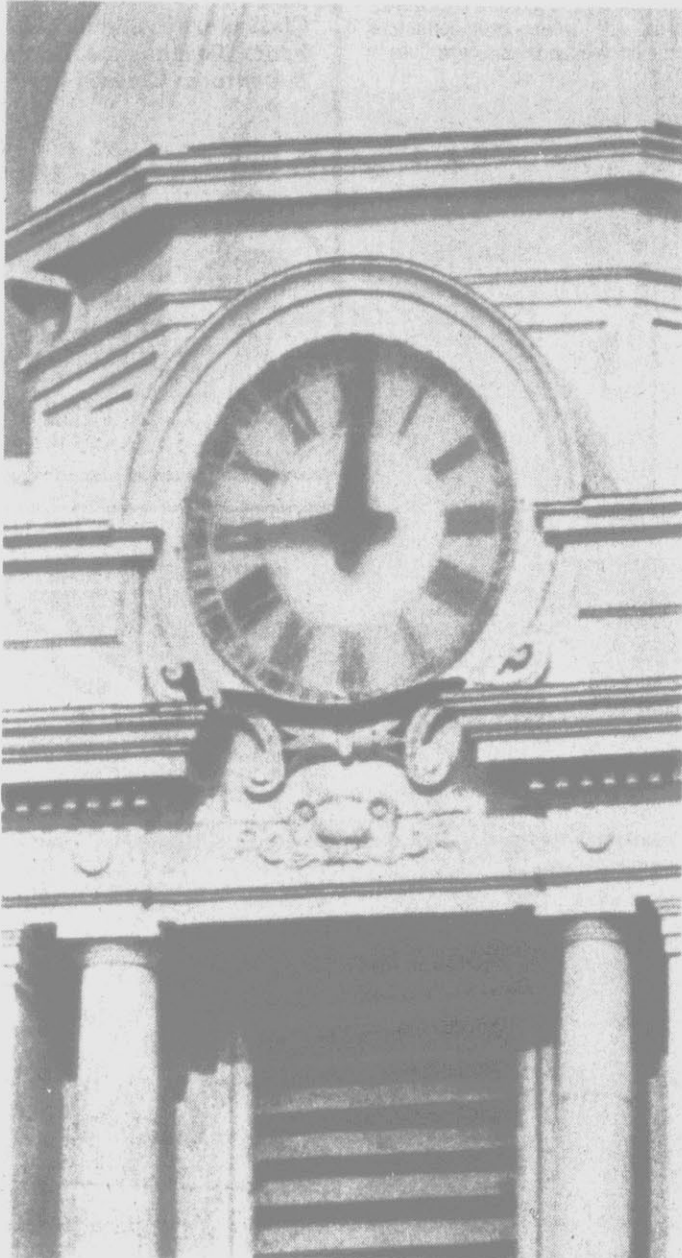
TIME FLIES — A passing bird takes time to look over downtown Greenville from its view on the ledge of the Pitt County Courthouse, ignoring the clouded face of the clock behind him. Weather has taken its toll on the courthouse clock, long a landmark for Greenville, but county building and grounds inspector Walter Gould says a facelift is coming up. Gould said the county issues a contract annually to have the clock lubricated and washed free of debris. (Reflector Staff Photo)
