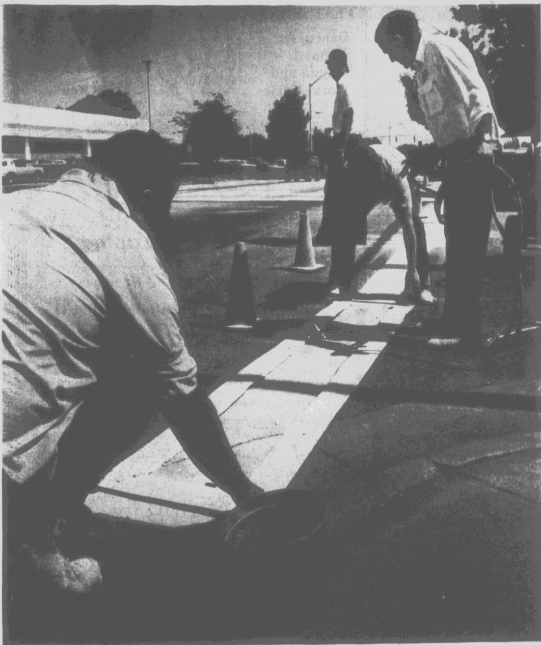
LINING THE STREETS — A Greenville road crew paints new lines at the corner of Greene and Second streets. The process involves stenciling lines or arrows on the pavement, painting with a quick-drying paint and
