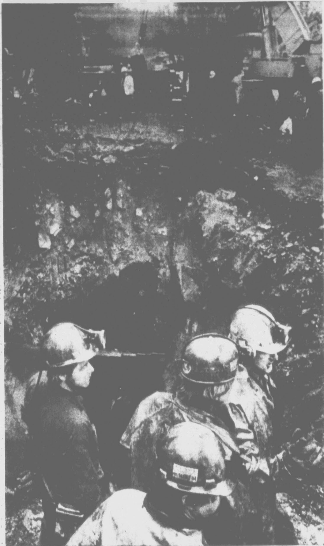
AIR SHAFT — Rescue workers, soaked in a steady rain, inspect an excavated air shaft to help in the search for five persons still missing after a car plunged into a mine hole near Llewellyn, Pa. One body has been
