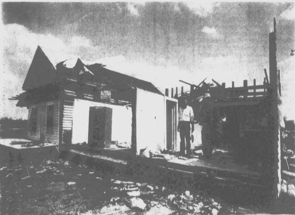
NOT MUCH LEFT — Lynn Haddock, left and Dean Girley stand in what is left of their house. Haddock said he and Girley were in the center of the house when the
