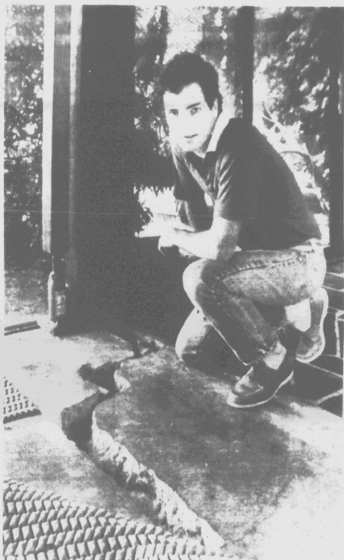
CRACKING UP — Ben Fleishman kneels by a four-inch crack in the floor of actor John Houseman's residence in Malibu, Calif., about 40 miles northwest of downtown Los Angeles. The Houseman home and 12 others have been declared unsafe by Los Angeles County engineers who ordered evacuation. The land on which the 13 homes sit is moving towards the sea at a rate of 1 1/2 inches per week. (AP Laserphoto)
