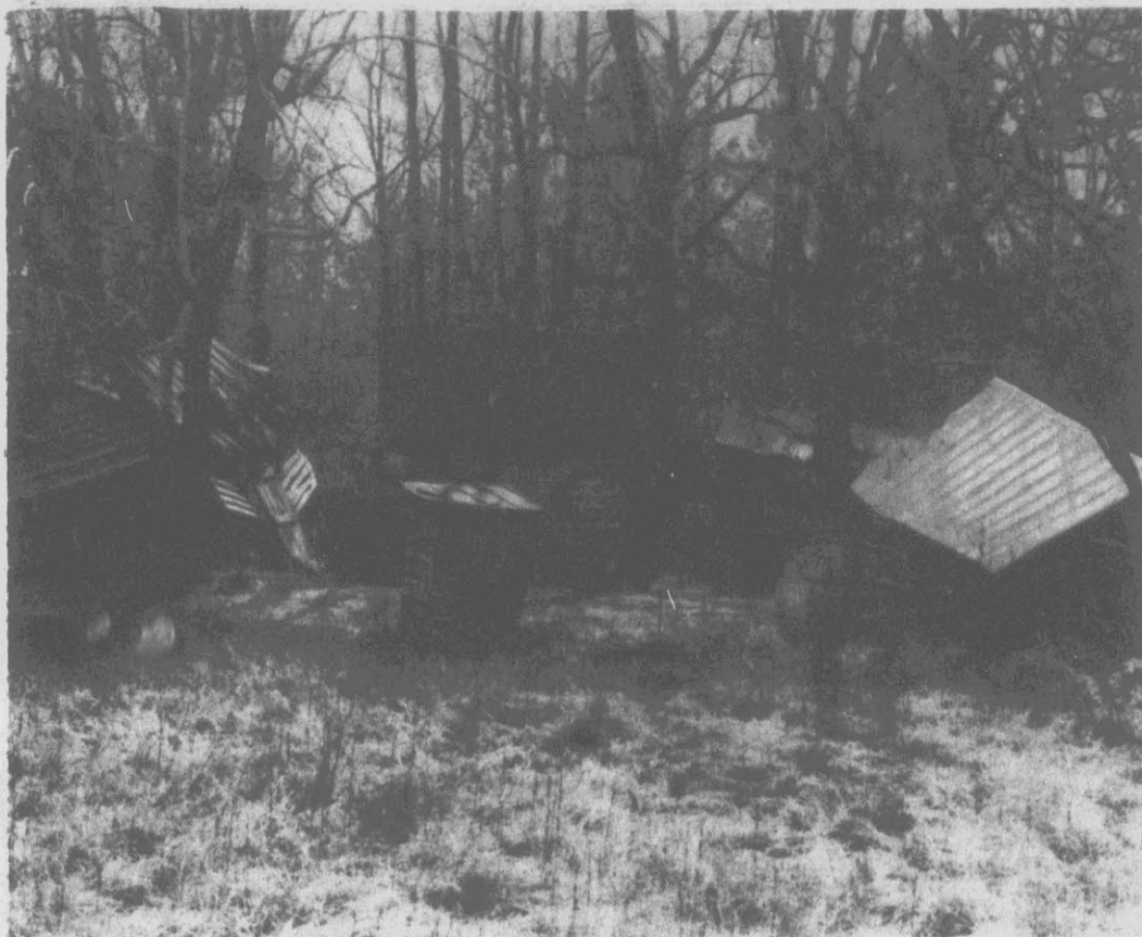
NEEDED — A TOUCH OF REPAIRS — This group of buildings along a roadside between the community of Shine and Goldsboro is in need of repairs to correct the altered states into which they have fallen into over the past years. One curious thing about this cluster of buildings — each is leaning in a slightly different direction. The group also calls to mind the raptures of nostalgia which songwriters and poets have often expressed for the remembrance of that tumbled-down shack back home. (Reflector Photo by Jerry Raynor)
