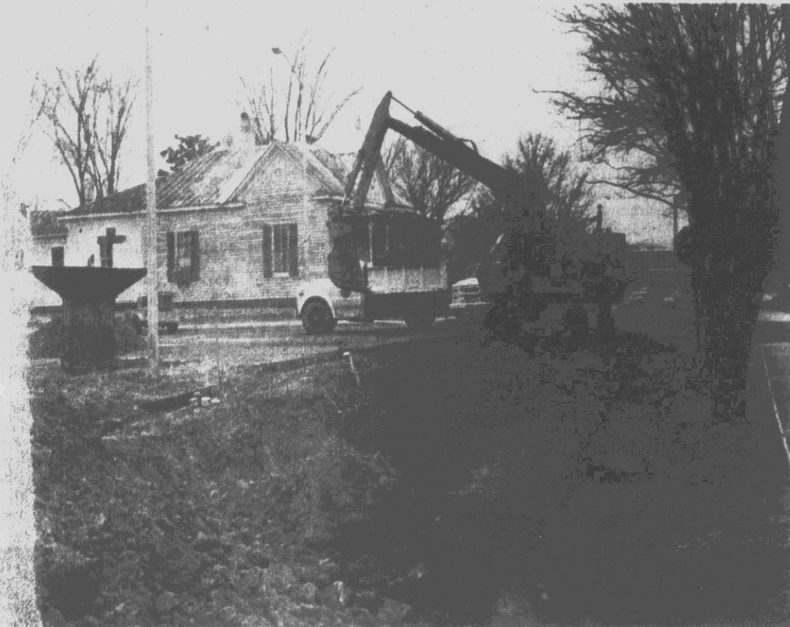
REPLACING SEWER LINE — Greenville Utilities Commission workers were in the process of replacing an 8-inch sewer line on Eighth Street, between James and Cotanche streets, today. Buzz Smart, distribution engineer for GUC's water and sewer department, said Cotanche Street would be blocked until the work is completed — probably today — and said the new line is replacing a line installed "at the turn of the
