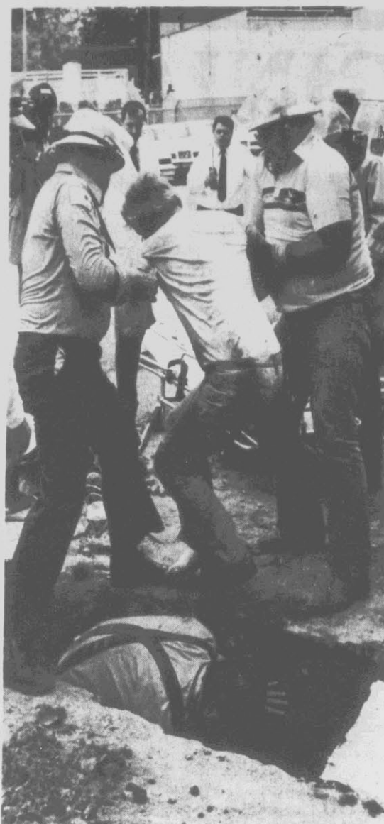
OUT AT LAST — Randy Edwards is helped from the ditch after a cave-in trapped Edwards and fellow worker Clarence Whitehurst Wednesday afternoon. Neither man was seriously injured during the ordeal. Fire/Rescue personnel worked for about four hours to free the two men. (Reflector Photo by Tommy Forrest)
