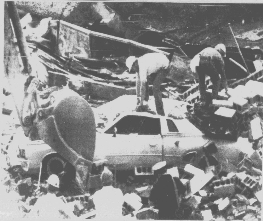
COMBING THE RUBBLE — Workmen stand on top of a car to remove rubble after a natural gas explosion ripped through a grocery store in South
