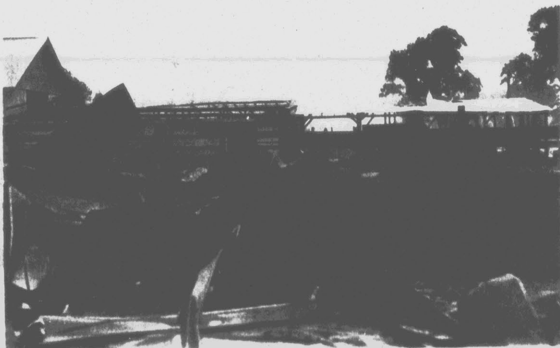
STORM DAMAGE ... Pieces of barn roof lie scattered about at Ram Horn Stables after the roof was ripped off 12 horse stalls by what
