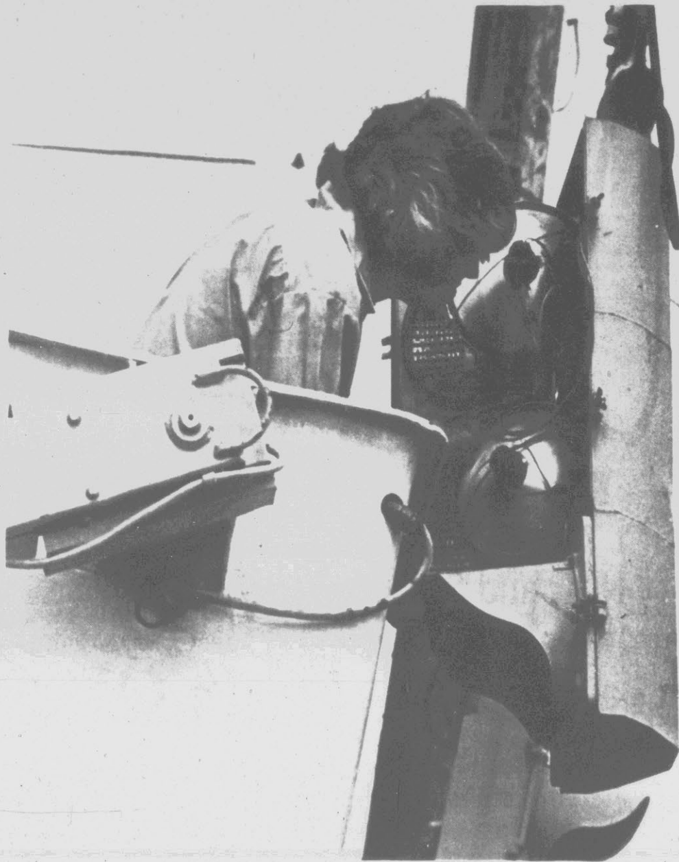
REFURBISHING STOP LIGHTS — Tim Nelson of the Public Works Department's sign and signal division makes wiring connections on a stop light in downtown Greenville this week as the department replaces stop lights with freshly repainted
