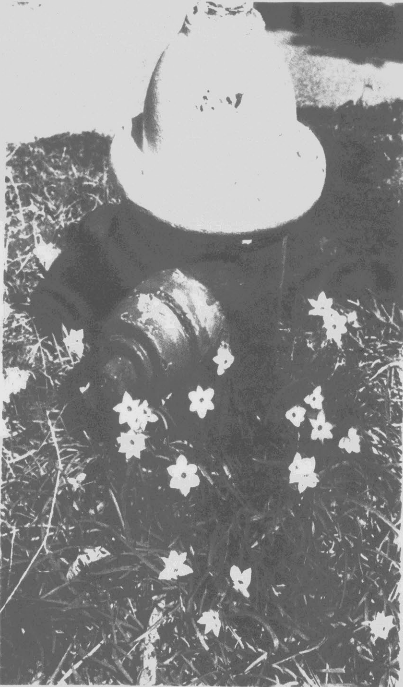
SPRING COMES TO A FIRE HYDRANT — Adding a new touch of color to the red and yellow of the hydrant. (Reflector Photo by of a short fire hydrant in Robersonville, Jerry Raynor)
