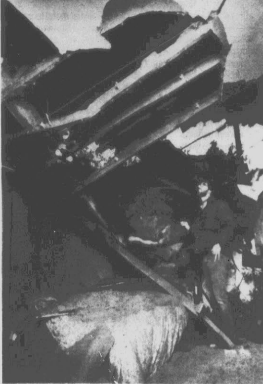
TREE DESTROYS BEDROOM — Pell Fender looks at his demolished bedroom after a tree fell on it during a storm in Menlo Park, Calif., Wednesday afternoon. No one was injured. Shrieking winds and pounding rains pummeled Northern California Wednesday, knocking out power, shutting down the Golden Gate Bridge and toppling trees. (AP Laserphoto)
