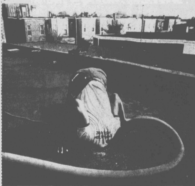
HELLO DOWN THERE — This photo does not show a giant worm carrying off a workman through a hole in the roof of a Philadelphia home. But it does show an insulation mechanic checking with a co-
