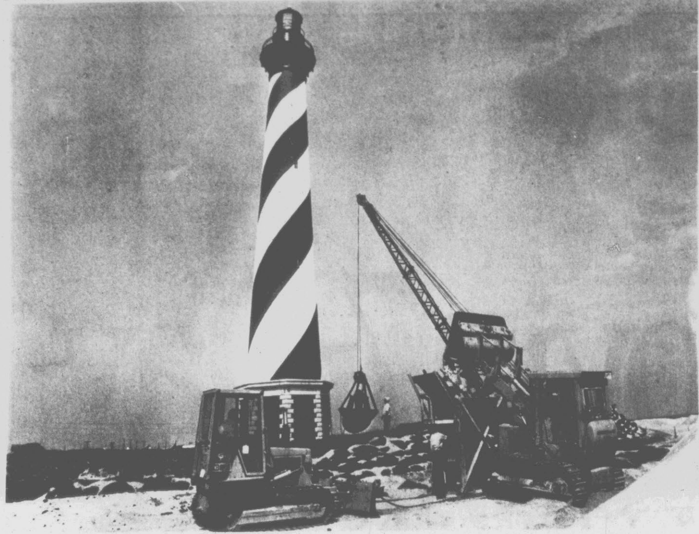
SAVE THE LIGHTHOUSE — Workers last week put the finishing touches on a wall of sandbags around the base of the historic Cape Hatteras Lighthouse. The work, financed by contributions, is part of a project to save the historic structure from destruction by the waters of the Atlantic Ocean. John F. Minges, chairman of the Save Cape Hatteras Lighthouse Committee in Pitt County, said Pitt is one of the top 25 counties in the state in the percentage of its county goal.
