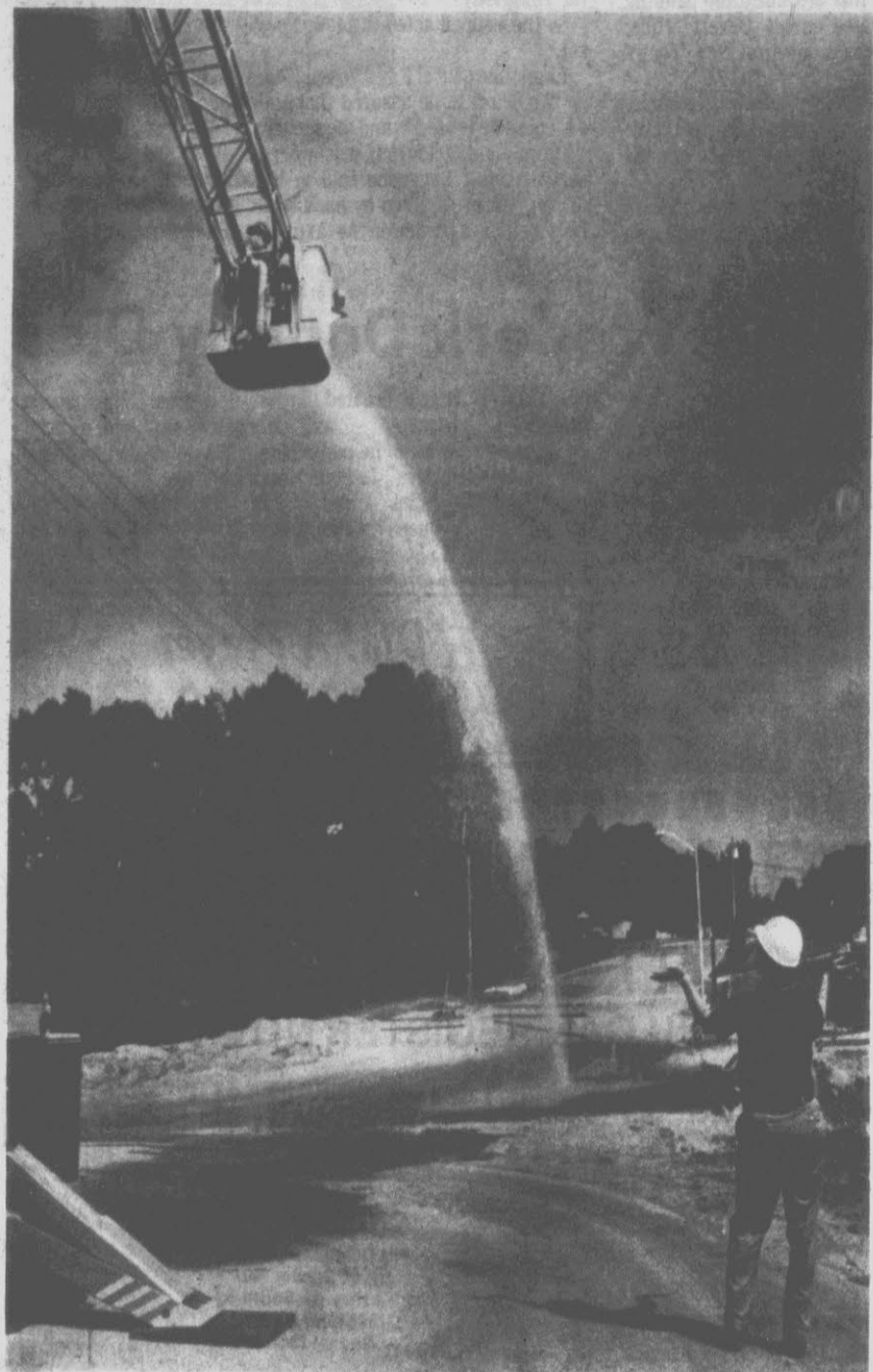
Greenville Fire and Rescue personnel pour a steady stream of water on the recently filled hole on First Street to show, according to Greenville Public Works Director Mayo Allen, where the weak spots are. Allen said the street, opened to traffic Friday, will remain unpaved for 30 days or "until we see just where trouble spots, if any, are located." (Reflector Photo By Mary Schulken)
