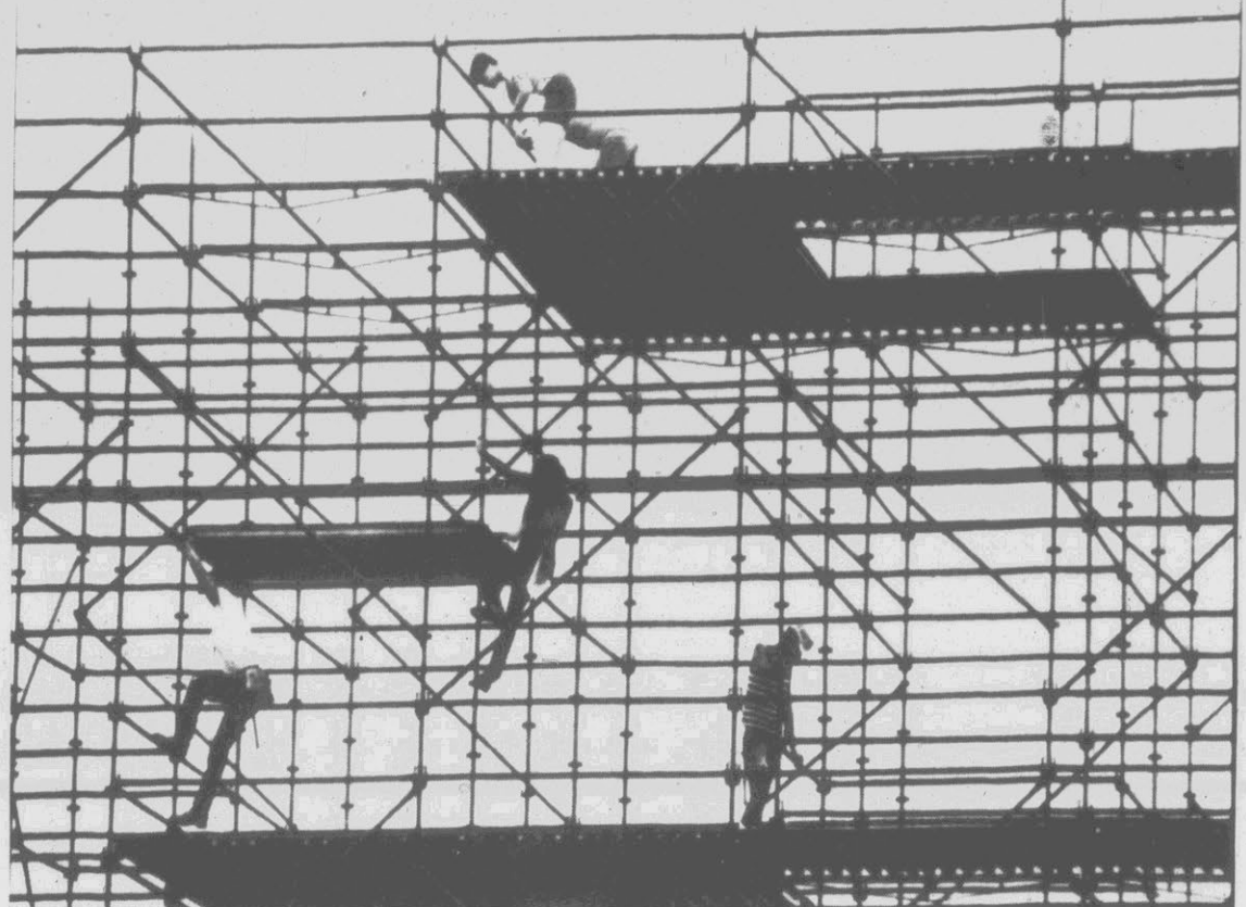
PREPARING FOR ROCK FESTIVAL — Workers ready the scaffolding around the stage as preparations continue for this weekend's UNUSON rock festival. It will be held in Glen Helen Regional Park north of San Bernardino. (AP Laserphoto)
