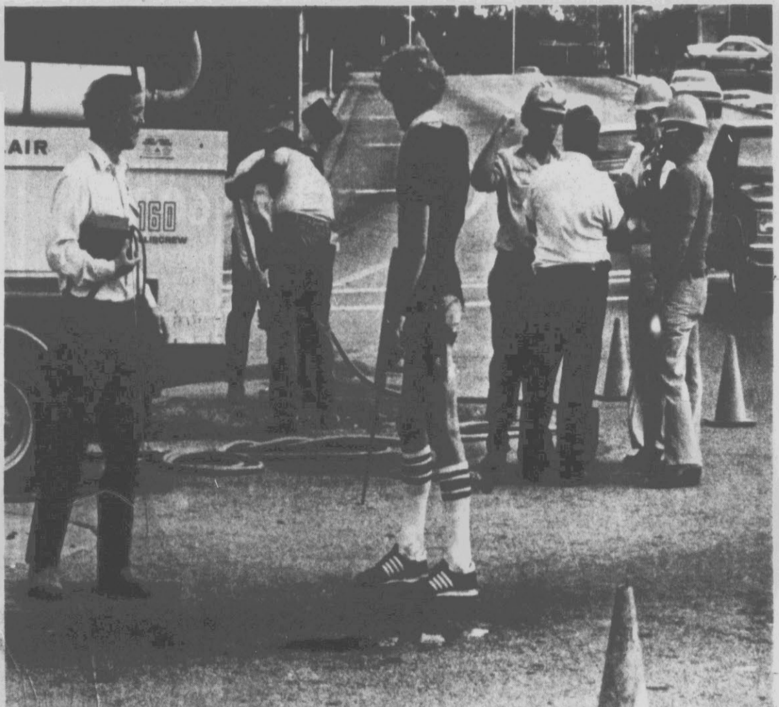
ON THE SCENE ... Workmen from the gas department of Greenville Utilities and others from a private firm converged at the intersection of Cotanche and Reade streets last Friday. A gas leakage had been detected at the site during an annual survey of the city's 43 miles of gas mains. Work has now been completed in locating and repairing a rusted main. Gas was leaking from the main, one installed at the site in the early 1900s. (Reflector Photo by Jerry Raynor)
