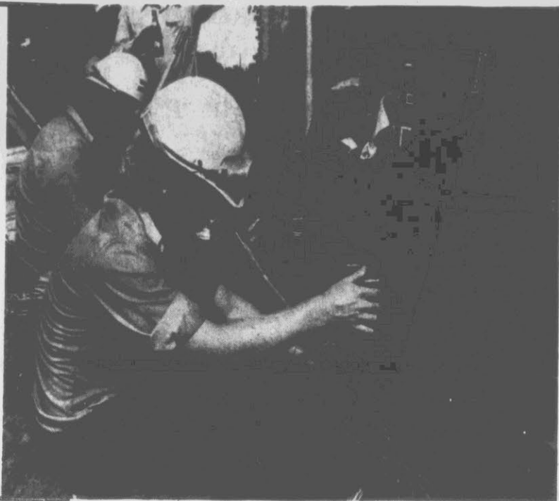
TERMINAL — Greenville Utility workers Ricky West, front, and Johnny Council wire an electrical terminal on the west side of the large hole Tuesday, in preparation for restoring electrical service. (Reflector Photo by Tommy Forrest)
