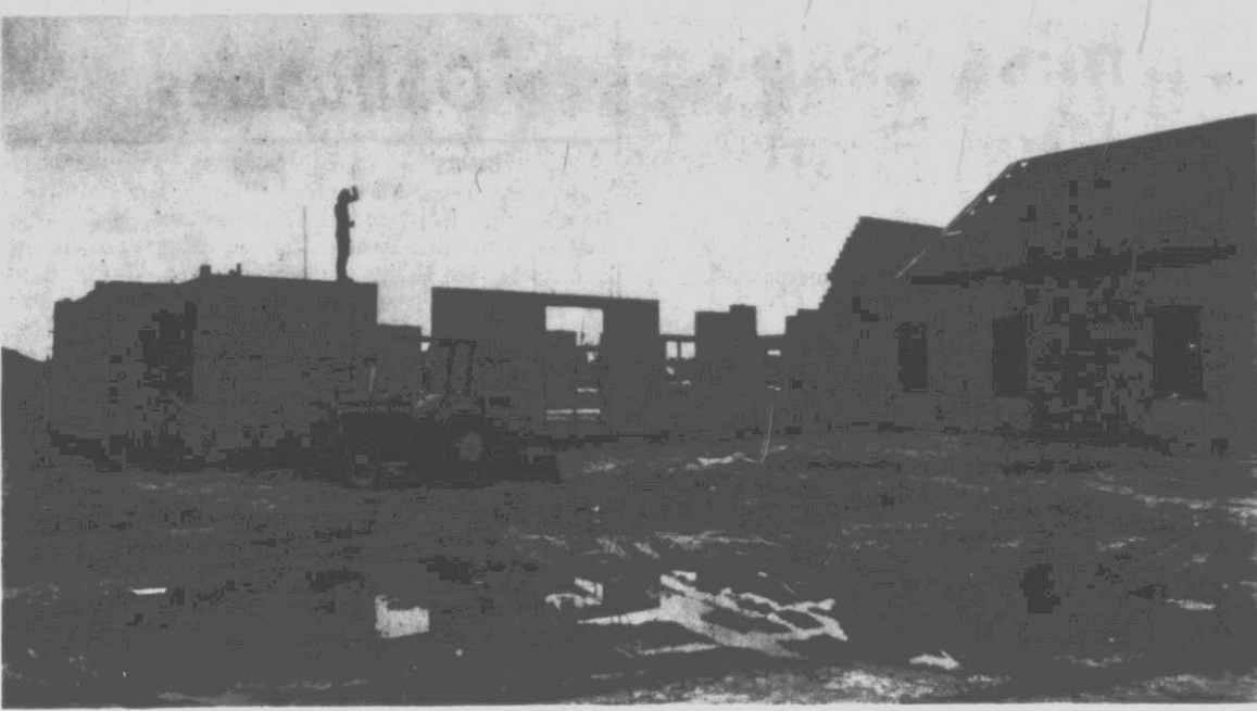
NEW CHURCH UNDER CONSTRUCTION — The Winterville Free Will Baptist Church is under construction on Cooper Street in Winterville. The church will be built in four phases, with the first stage slated for completion in June. (Reflector Photo by Tommy Forrest)
