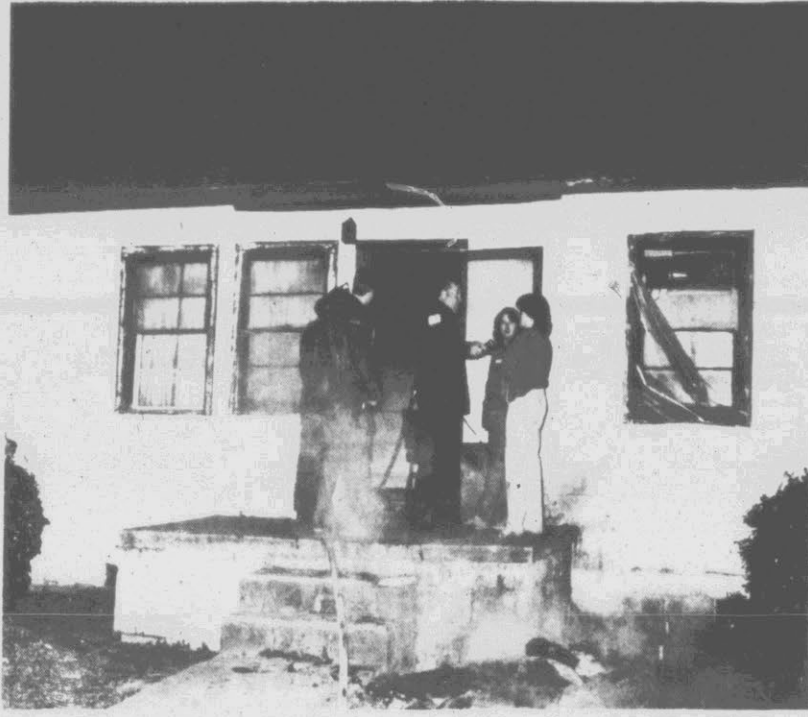
MODERATE DAMAGE TO HOUSE — Greenville fire-rescue officials look over a house that was damaged by fire Thursday night. According to records, the house was occupied by Danny Braxton and the owner was listed as Woodrow Haddock. The house, which is located off Evans Street Extension, received moderate damage during the blaze. Cause of the fire was under investigation. (Reflector Photo by Tommy Forrest)
