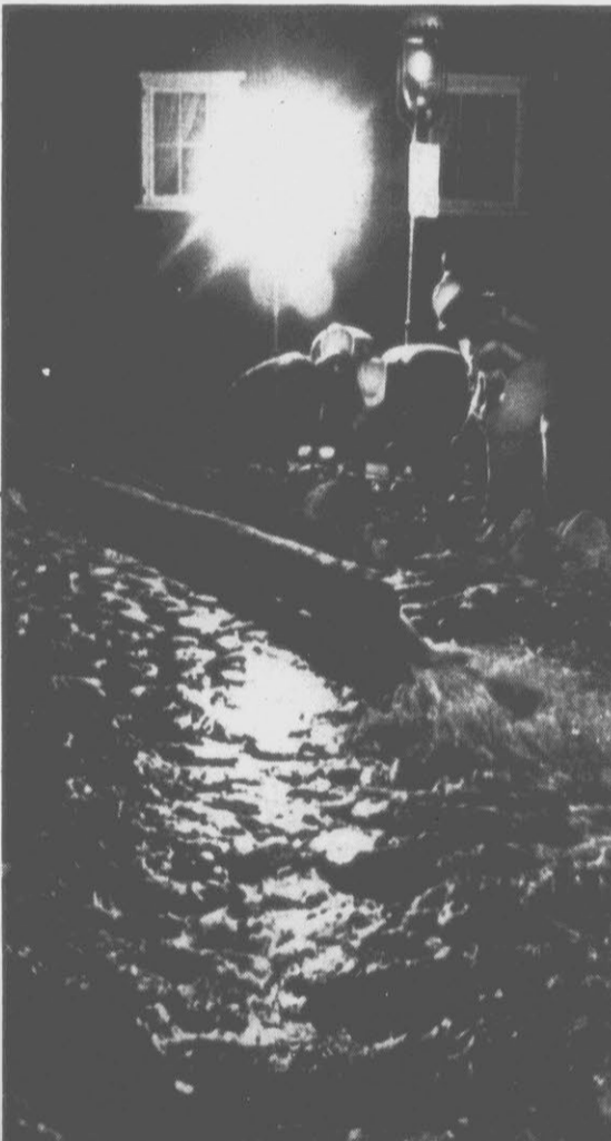
BROKEN WATER MAIN — Workers dig through the cobblestones of Chalmers Street Saturday night to get to a broken 24-inch water main serving parts of downtown Charleston (S.C.) and James Island. The break was caused by the change in temperature from cold water coming from the Edisto River 60 miles upstream and the relative warm weather Charleston had on Saturday, according to a spokesman for the Commission of Public Works. (AP Laserphoto)
