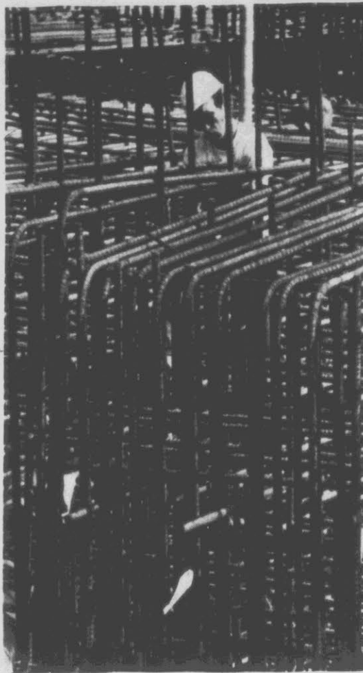
FOREST OF STEEL — A hard-hatted worker is surrounded by a forest of steel as he works at Space Launch Complex 6 at Vandenberg Air Force Base in California, future West Coast home for the space shuttle. (AP Laserphoto)
