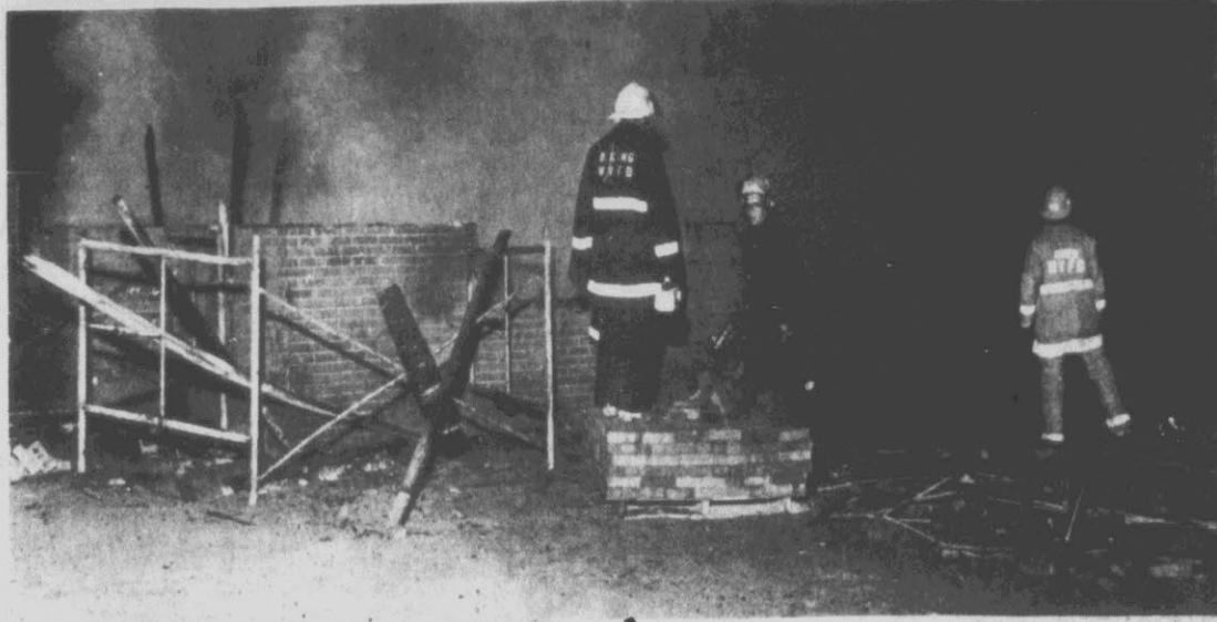
FLAMES DESTROY APARTMENT — Ayden and Winterville firemen look over rubble left after flames destroyed an apartment under construction on Liberty Street in Ayden Wednesday. Firemen arriving on the scene found the duplex fully involved with fire. Officials said the apartment is part of a federal housing project under construction by Site Construction Co. Damage estimates were not available. (Reflector Photo by Tommy Forrest)
