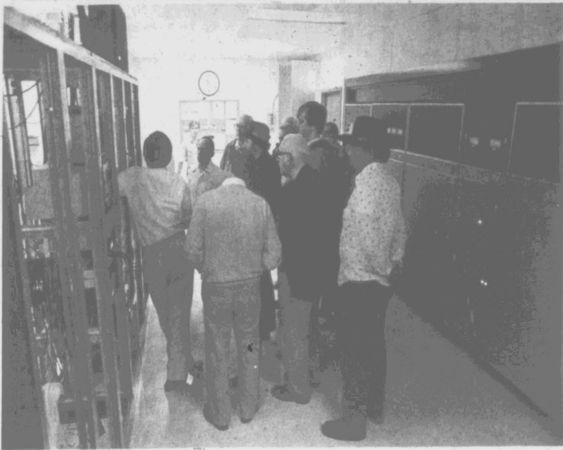
NEW TRANSMITTER IN OPERATION — Members of the Brightleaf Amateur Radio Club get a tour of the new WNCN television transmitter at Grifton Tuesday night. Station engineer Macon Dail (with back to camera, far left), describes some of the new equipment to the club members. The new RCA transmitter, which is a state-of-the-art model, is shown on the right. The new facility replaces the older transmitter that had
