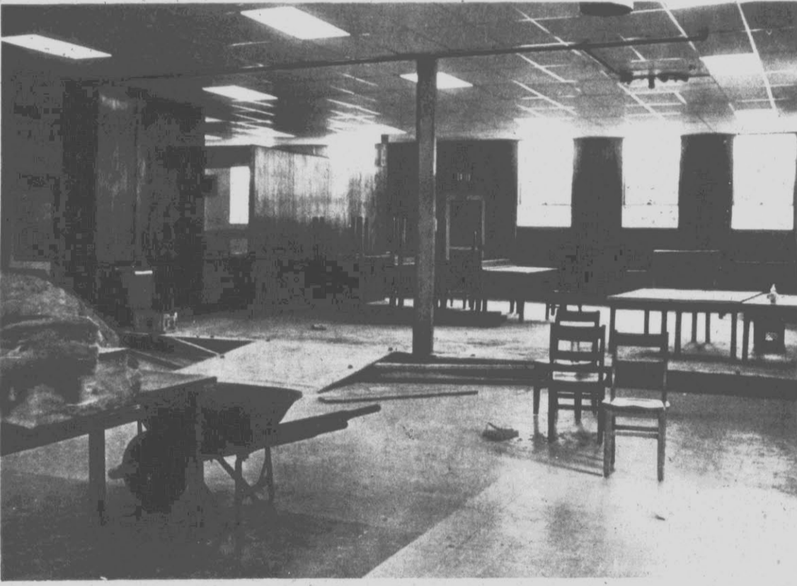
LUNCHROOM ENLARGED AT STOKES . . . Stokes Elementary's lunchroom facilities were enlarged by closing in part of the gymnasium and converting it into an eating area. The addition doubled the eating area. (Reflector Photo By Mary Schulken)
