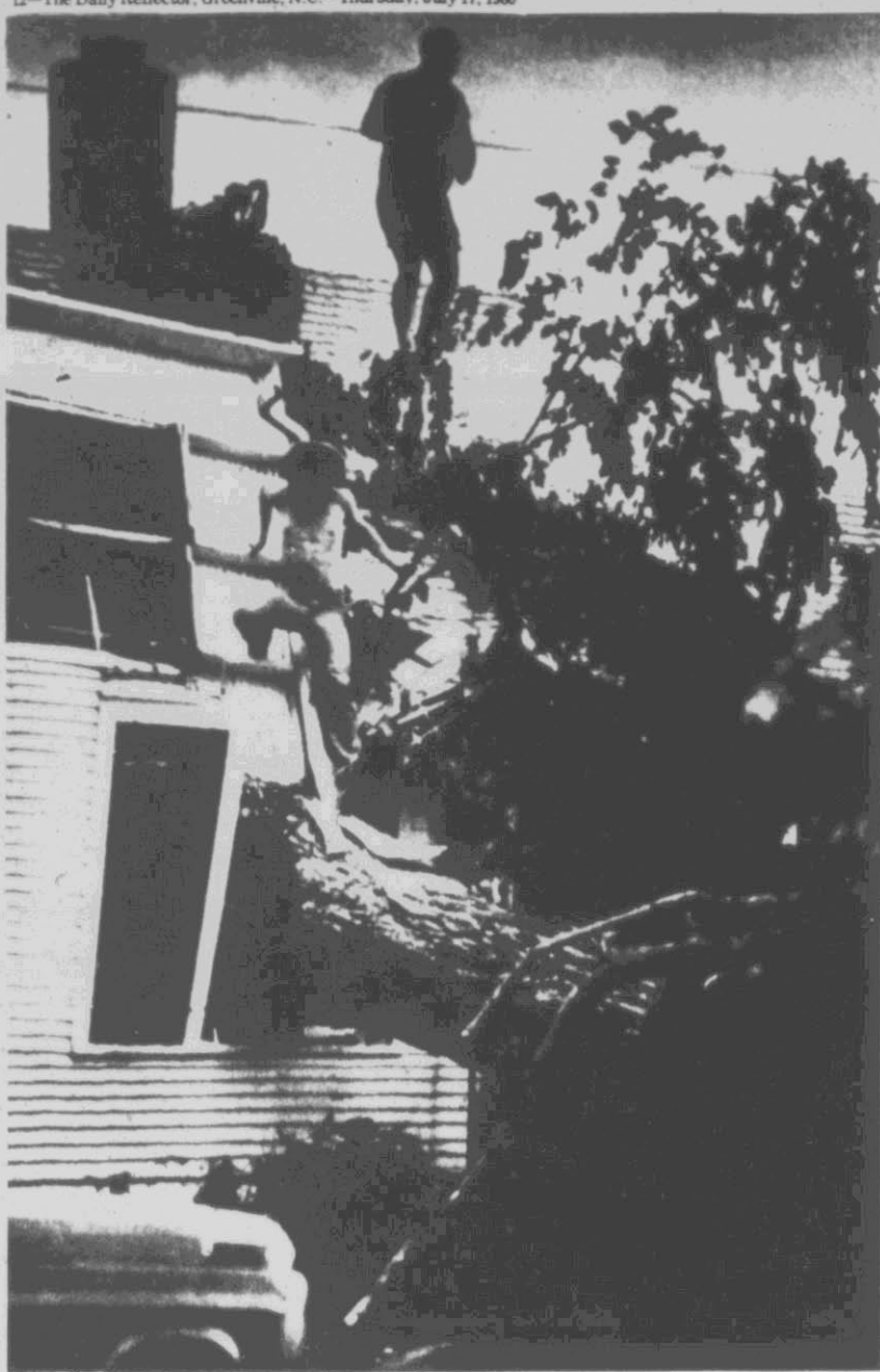
COMPLETELY THROUGH THE ROOF — This home in a residential section of Eau Claire, Wis. was almost sliced completely into two sections when a tree toppled by night winds went through its roof. One occupant inside narrowly escaped serious injury and
