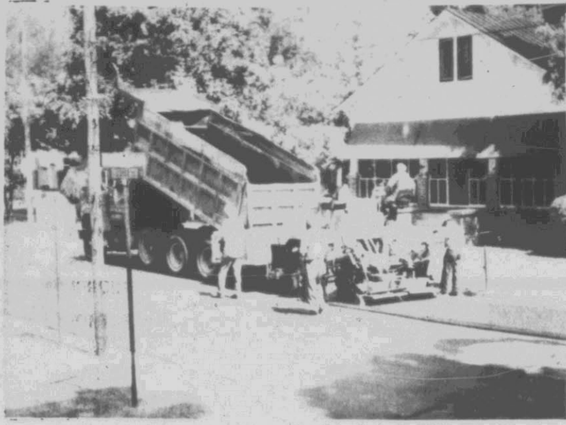
RESURFACING COMPLETED... Workmen place a new layer of asphalt on a section of 13th Street near Forbes Street recently as the city completed its program of local resurfac-
