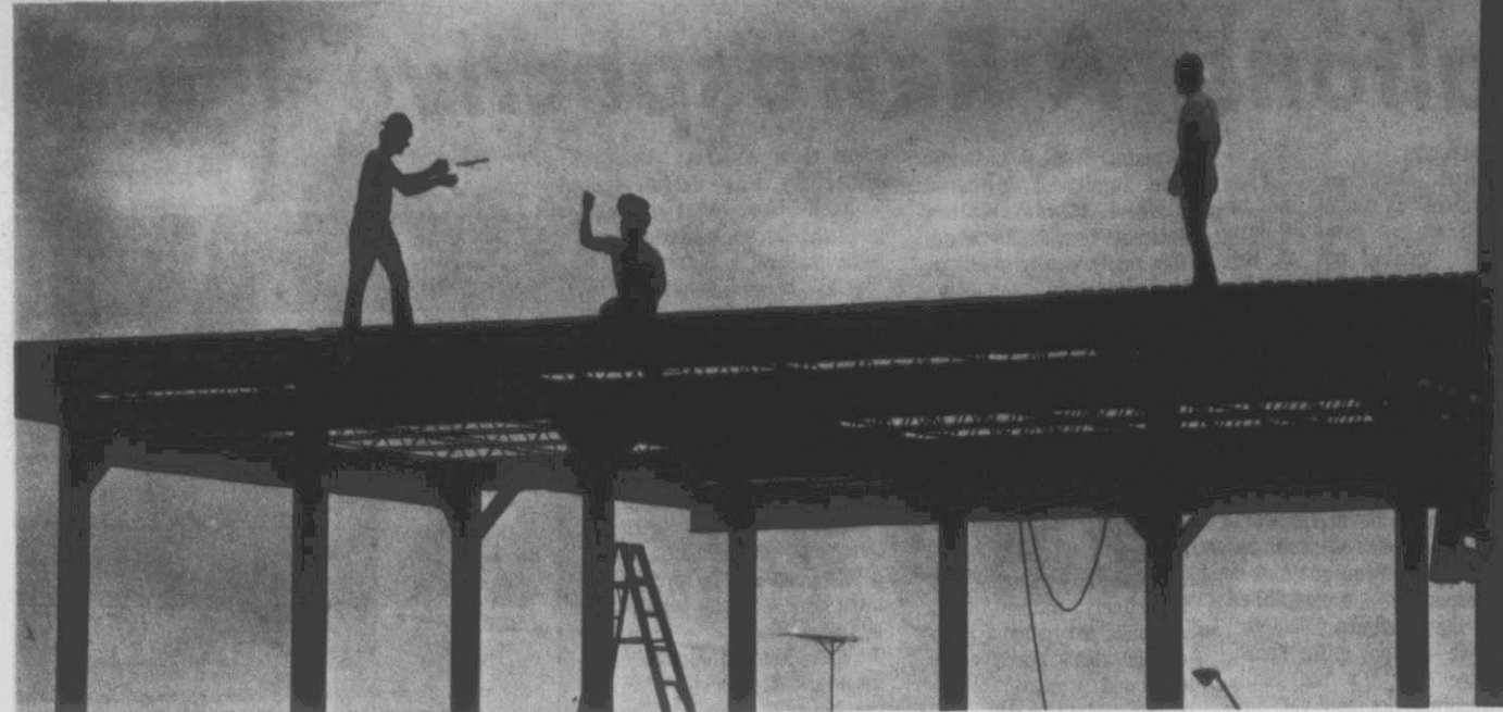
ON TOP — Workmen atop the new North State Savings and Loan, at Second and Washington Streets, are silhouetted against a partly cloudy sky as they proceed with the day's work. (Reflector Photo by Tommy Forrest)
